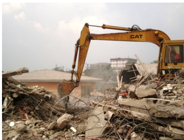
Figure 10. Collapse site of a 5-storey building at Nkoldongo, Yaoundé (Source: Journal du Cameroun, 2010)
