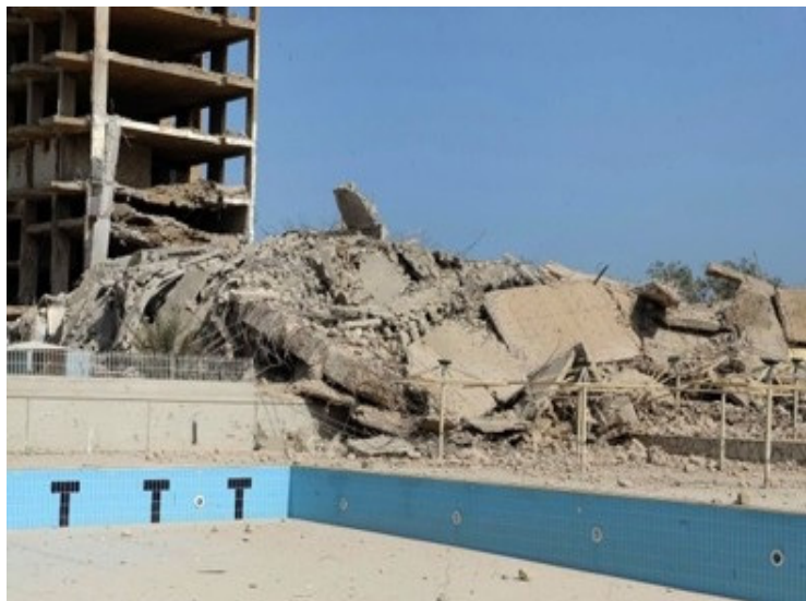
Figure 8. Collapse site of a 4-storey building at Akwa Nord, Douala (Source: Journal le messenger, 2014)
