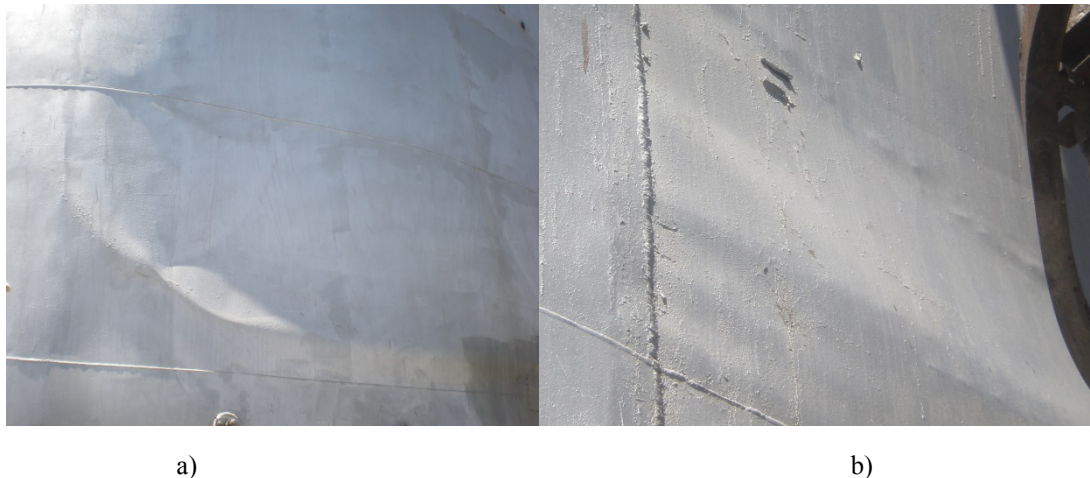
Figure 1. The form of the hollows on the wall of the standpipes in the zone of erection joint
