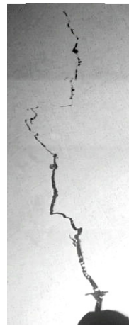
Figure 4. PD3 Static Load Crack
