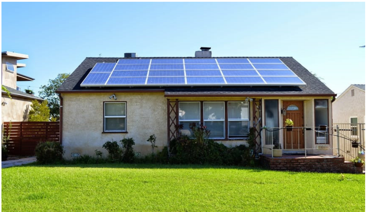
Figure 1. A home with rooftop solar in Los Angeles, California (divanov/Shutterstock.com)
