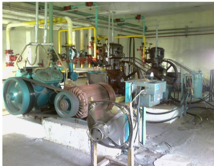
Figure 3. Compressor's room of a refrigeration unit in a cold storage
