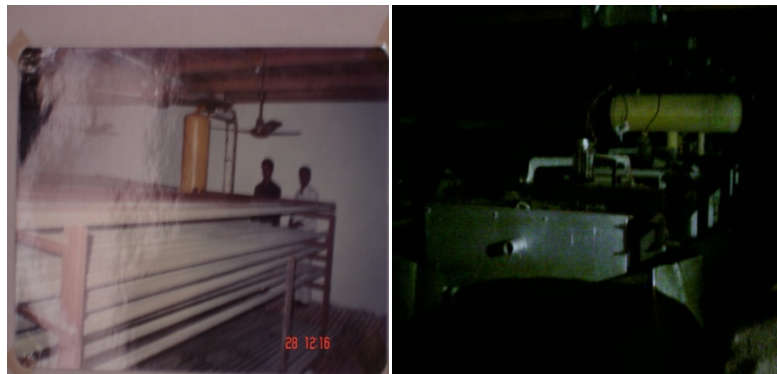
Figure 4. Air handling unit a) Banker type b) Fan coil unit
