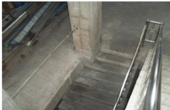
Figure 3. Stainless steel handrails on the fire escape stairways
