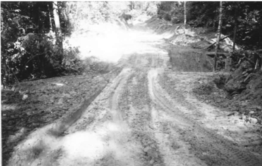
Figure 5. Road failure caused by insufficient crown opening
