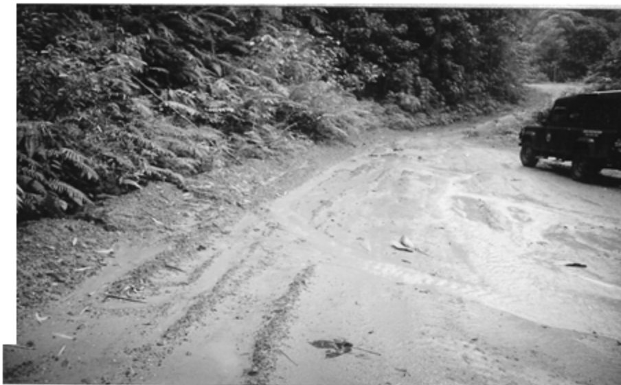
Figure 6. Consequences of improper maintenance of the side ditch caused water flow on road surface.
