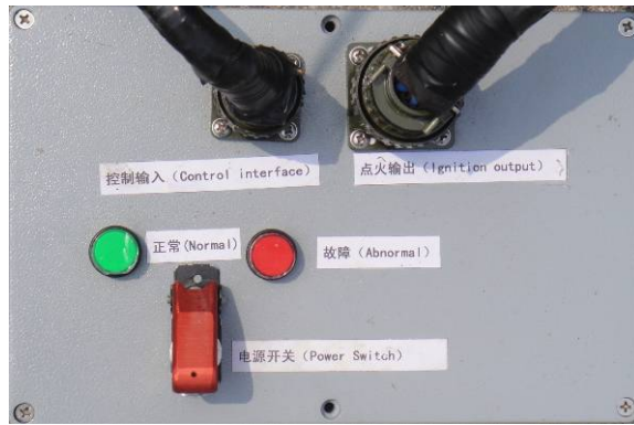
Figure 2. Main Control Box
